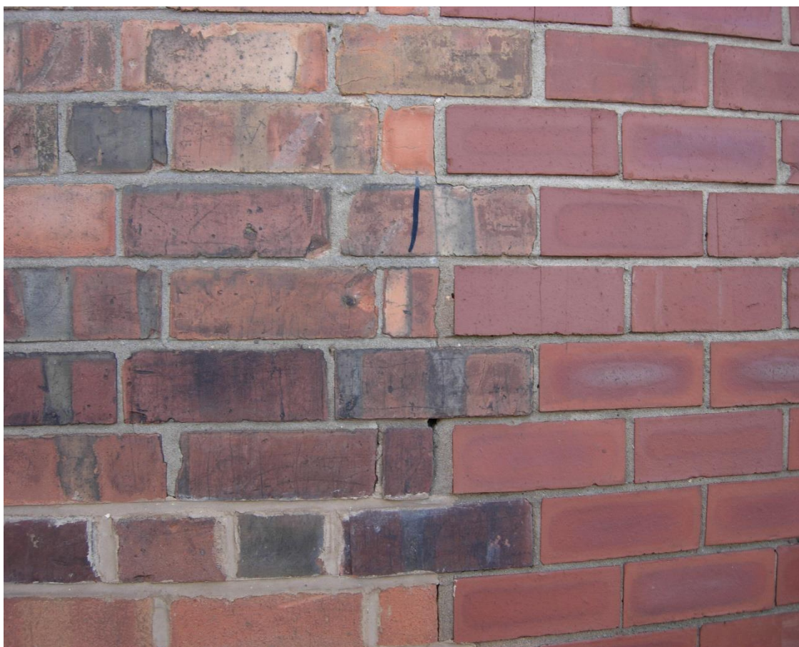
Photo 61: Repairs to brickwork do not match the older type and unsympathetic cement rich pointing that does not match the original mortar type and finish on older structures should be avoided.
